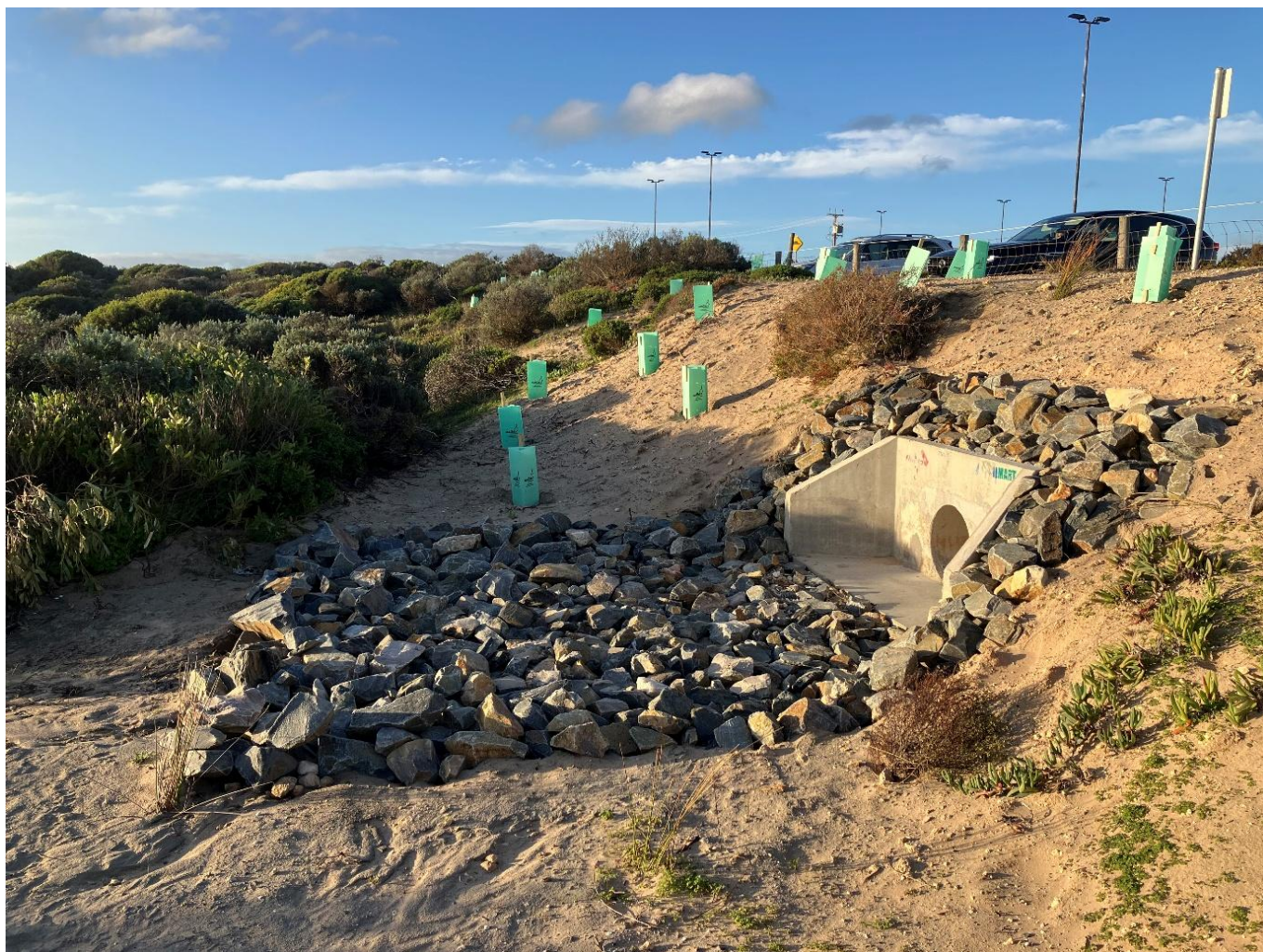
Stormwater outlet directing run off from the carpark at Beach Road into sand dunes, Goolwa (C Taylor)
