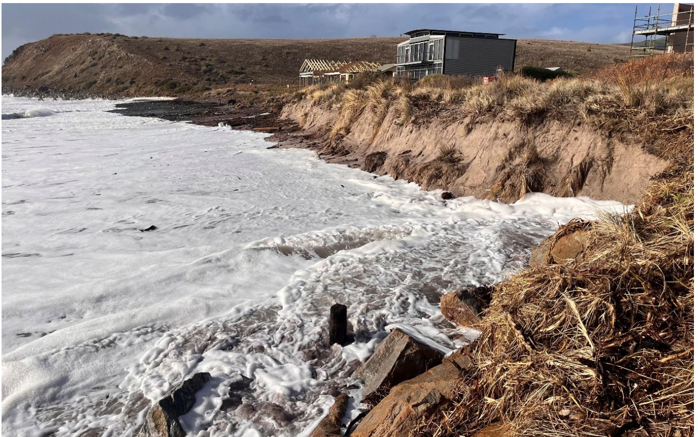
Impacts of storm erosion due to large storm surge and high tide event causing loss of several metres of dunes in July 2025 (Not contrast to image below) (C Jackson)
