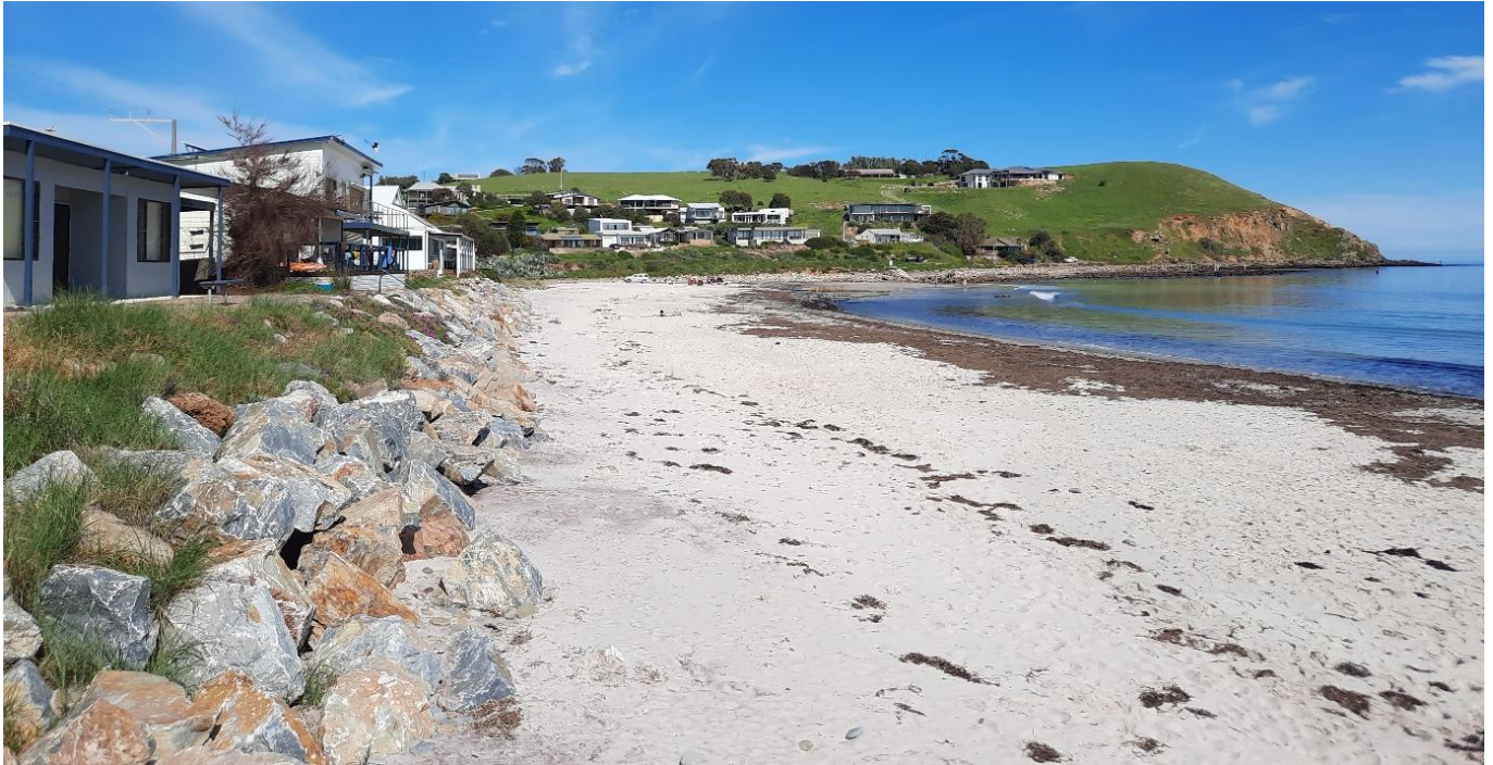
A private seawall in front of properties in very close proximity to the coast that often experience wave overtopping during storm events (S Sutherland)
