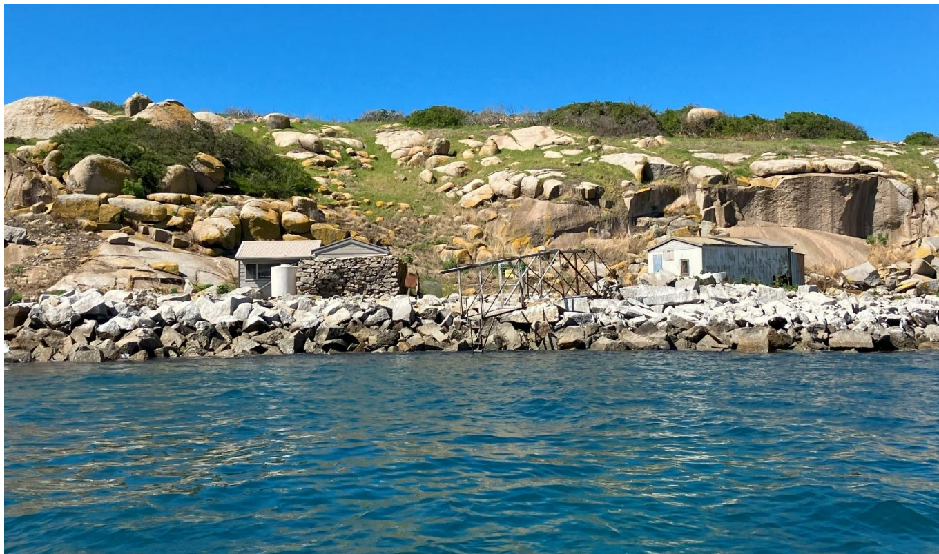
West Island research facilities and jetty structure require repair and maintenance (C Taylor)
