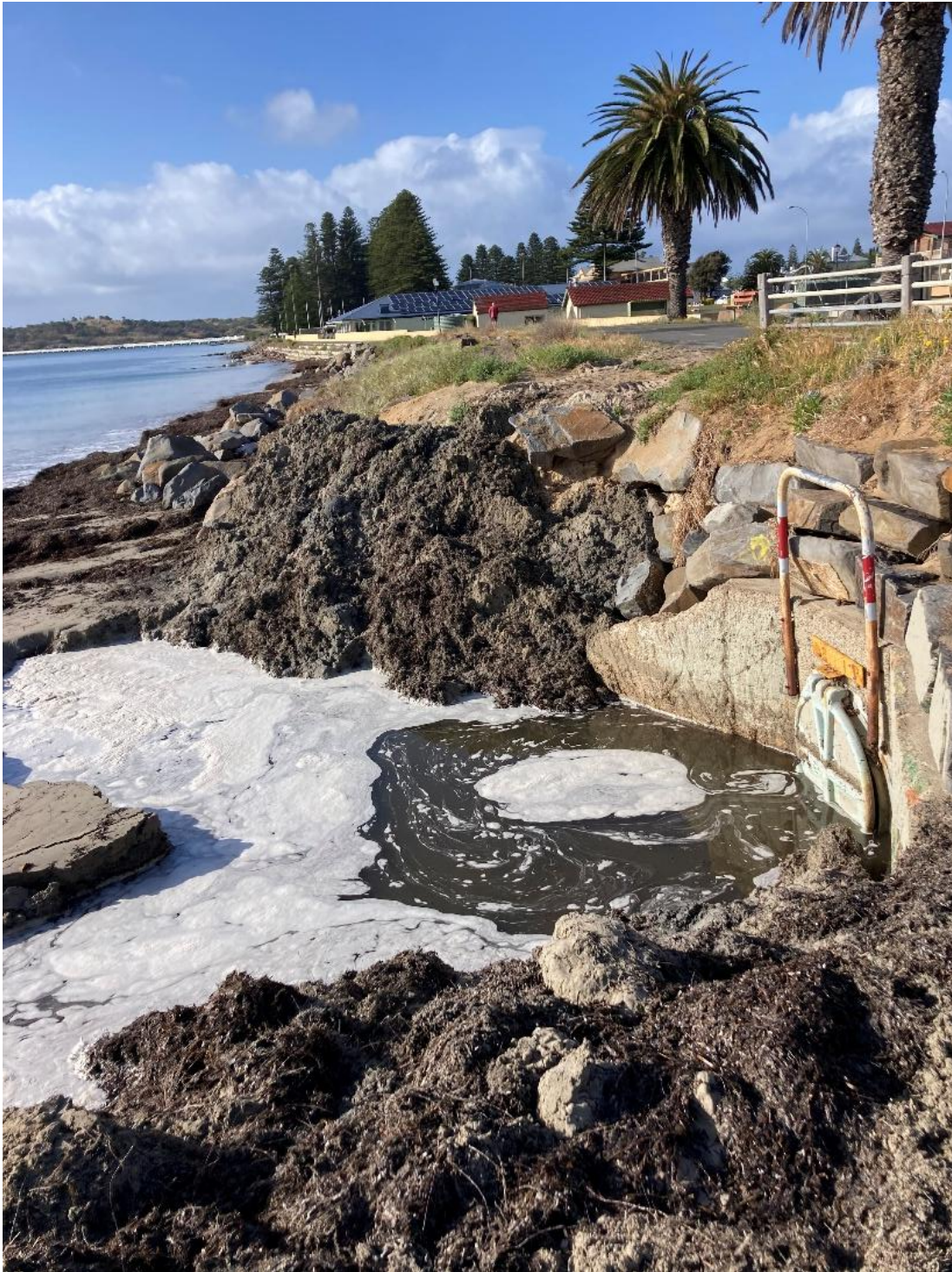
Stormwater outlets releasing directly onto the beach (R Shirlaw)
