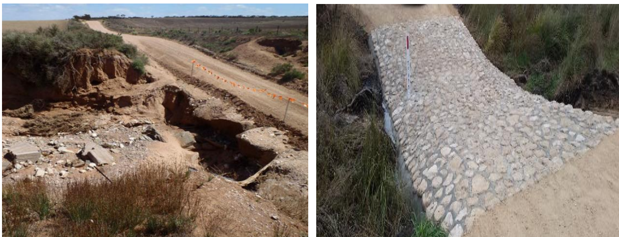
Figures 1 and 2: To the left is a failed ford crossing and to the right is a well-designed and constructed for crossing.
